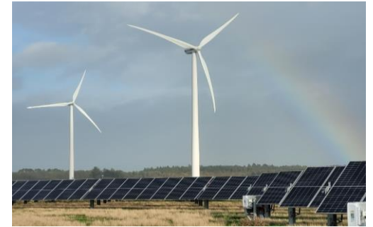
📷 1 Power generation facility in Holmen, Denmark, developed by EE
