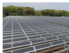
Tokorozawa Kita-Iwaoka Solar Power Plant
