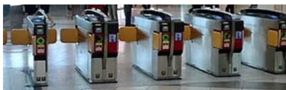
Automatic Ticket Gate lease to Kintetsu Corp.
