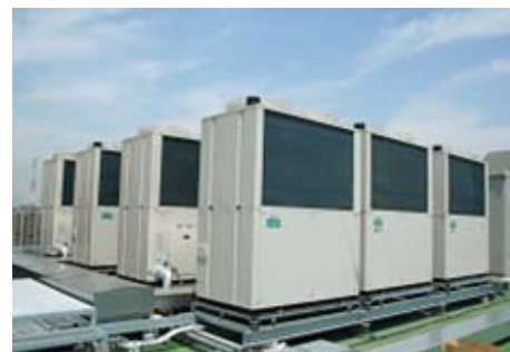
Chiyoda Corporation has introduced our ESCO to achieve energy saving.
