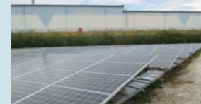
Solar power generation system (Saga Pref.)
