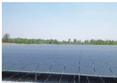
Solar power generation site
